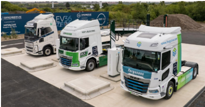
High-power charging facilities at the Sunderland Plant
