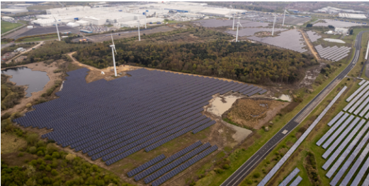
Solar power generation at the Sunderland Plant
