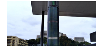
Solar cells installed on a canopy pillar
