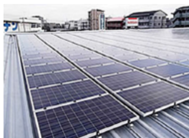
Solar panels installed on the roof of a Kanagawa Nissan dealership. Power from the panels is supplied to dealerships through the Nissan PPS system.
