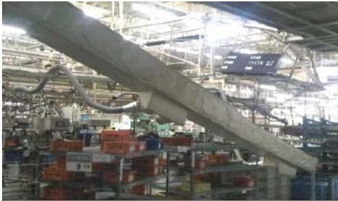
Collapse of air ducts
